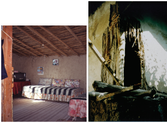
Figure 15, 16. Ridge roof construction without truss, and reed covering material. Adana, 2000 and Huğ House's wall detail, Mersin, 1998 (demolished in 1999)
