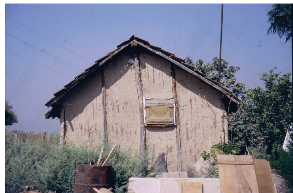
Figure 13. Side elevation of the registered Huğ House next to Mersin Yumuktepe Tumulus, 1998.
