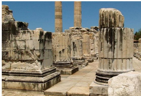
Fig. 12. Crack formation and deterioration of stone blocks in a historic temple structure
