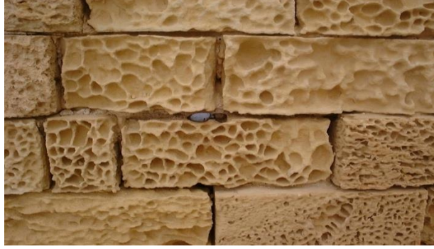
Fig. 1. Stone wall composed of blocks exhibiting signs of salt-induced erosion
