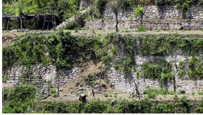
Fig. 9. Deterioration of dry-stone terrace walls in the Tramonti, Salerno region of Italy.
