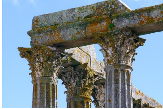
Fig. 2. Damage to a historic building caused by biodiversity loss and microclimatic changes.
